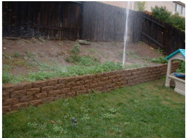
Broken Sprinkler head, causes "geyser". pressure loss does not allow other heads on the zone to function.
