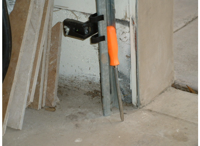
Photo-electric sensor for garage door is more than 6" above the floor and is a child-safety hazard.
