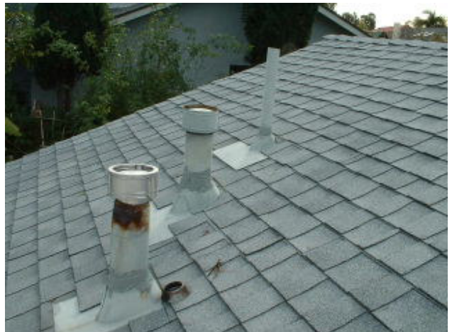
Furnace vent was nearly corroded through. // Storm collar was off of plumbing vent stack. Heater vents missing storm collars. // Cement Asbestos (Transite) water heater vent in middle.
