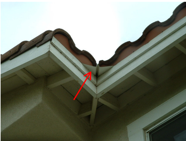
Valley flashing is 22" wide. The flashing should extend out from under the tiles and over the edge of the fascia. Only about 6" width is visible. Will lead to water damage at Eave.
