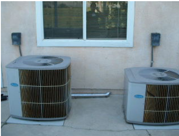
Concrete walk was poured around base pads of A/C units. Units should be elevated 3" above grade. // Units not secured in place. // Right electrical box behind unit.
