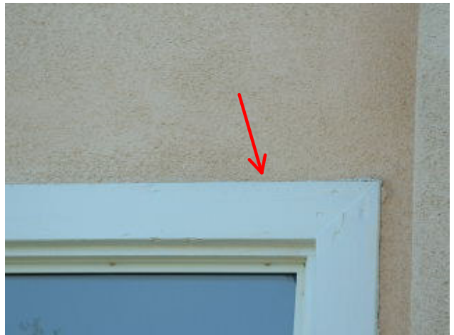
4 year old house: Missing drip cap flashing at exterior above window. Resulted in water intrusion at interior.
