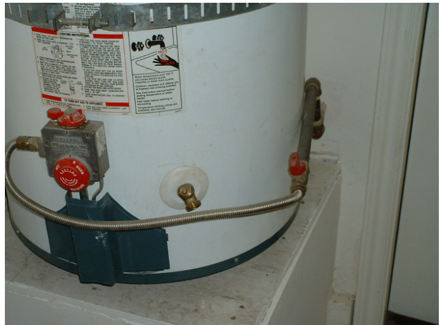
Water heater installed against gas pipe. Strained gas pipe. // No overflow pan.
