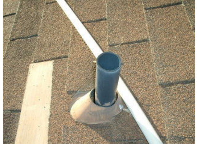
Improper flashing at plumbing vent stack. Wrong size jack. No storm collar.
