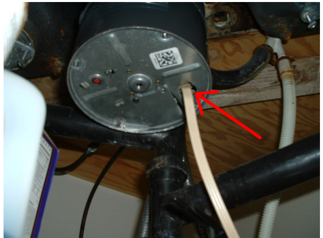
Missing strain relief cable bushing at disposal. Electrical connections can be pulled on.
