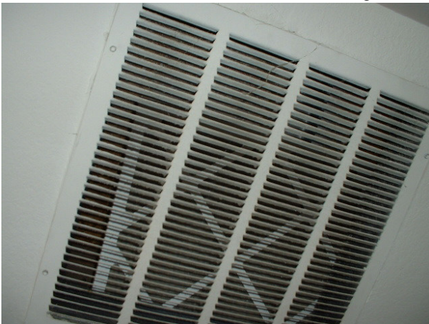
Filter inappropriately installed at a ceiling return-air grill where there is no filter provision. Filter is displaced because there is no retention system.
