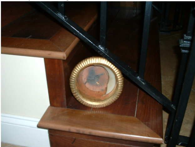
3 year old house. Improper railing construction. 6" sphere should not pass through triangle formed between rail, riser & tread. Child safety concern.
