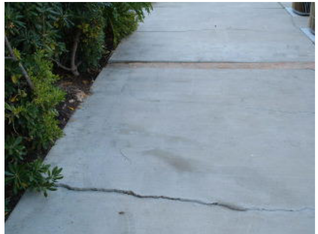
Cracks and uneven settlement in walkway are trip hazards.
