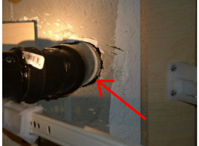
Wall under bathroom sink was not sealed at plumbing drain pipe penetration.
