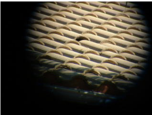
4 year old house: Example of a slipped roof tile from improper installation. More to come.
