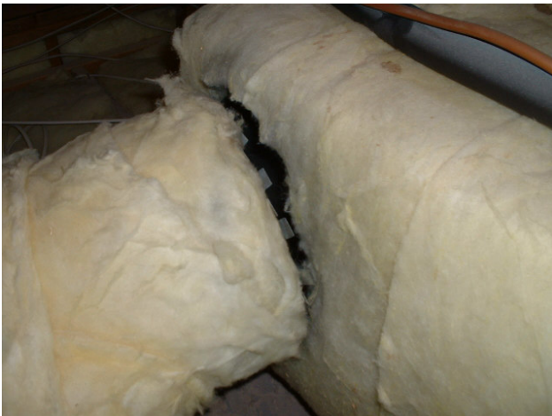
4 year old house: Improperly installed duct at air handler became nearly detached.
