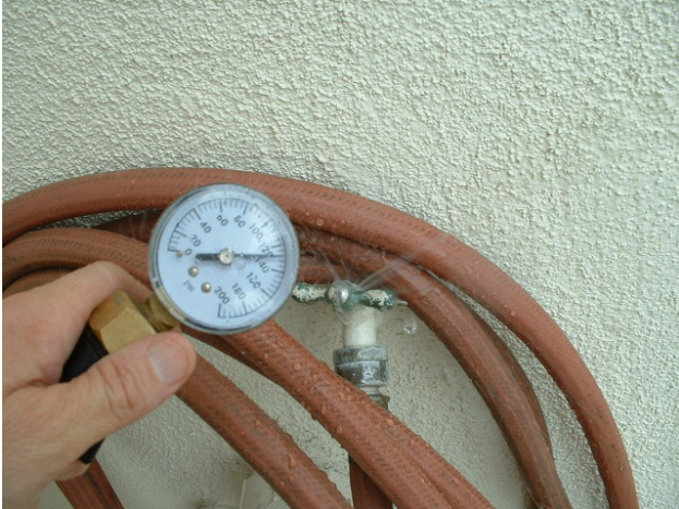
Excessive water pressure, nearly 130 psi. Valve stem leaks. No backflow preventer.
