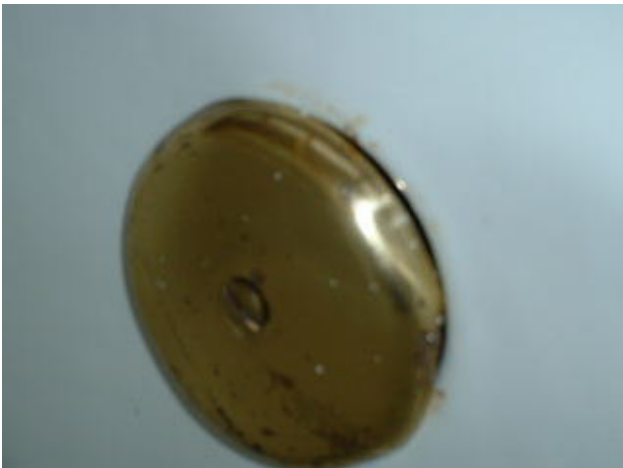
Loose & misaligned Tub overflow plate. Substantial potential for leaks.
