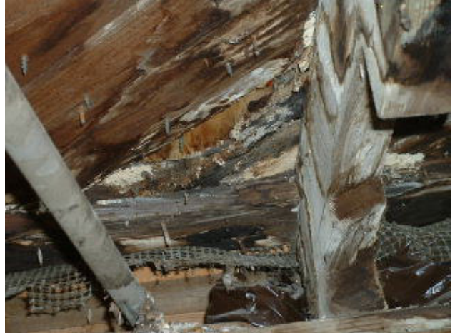
Mold damage under bathroom. Joist was cut away. Pest screen at crawlspace vent was damaged where pipe was run through.
