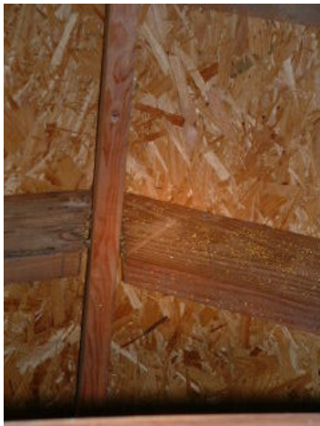
Rafters are separating from ridge board due to excessive structural movement.
