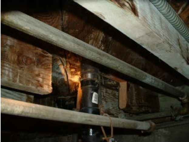
Moisture & mold damage unrepaired under bathroom. Old Galvanized plumbing present. Several Structural floor joists were inappropriately cut away.
