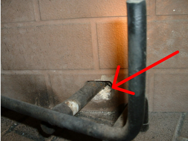
Missing fireproof grout at Fireplace wall. This needs to be sealed to prevent gas, fire, smoke & embers from entering wood structure. Minor repair.
