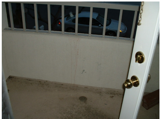
No overflow drain. // Short wall provides foothold for small children to climb up. While not a specific violation, common sense would dictate precautions.
