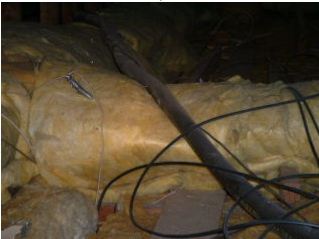
AC Refrigerant line set in attic was routed across and crushed Asbestos air duct.
