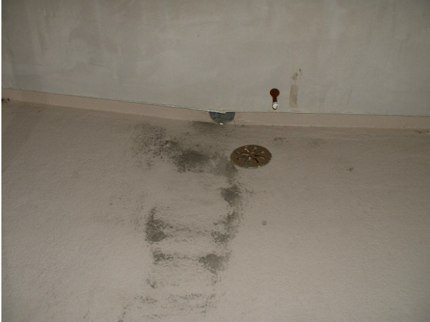
Overflow at deck is below primary. Water bypasses main drain and splashes onto walkway 2 stories below. Primary drains to street, but will not function properly.
