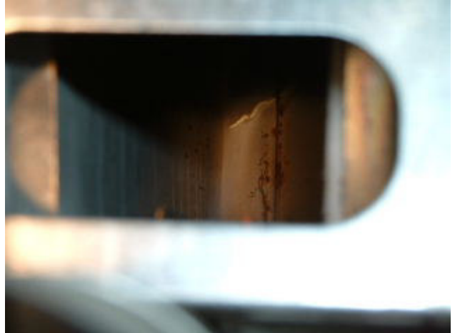
Cracked heat exchanger in Furnace. Life safety concern due to carbon monoxide. Furnace requires replacement.
