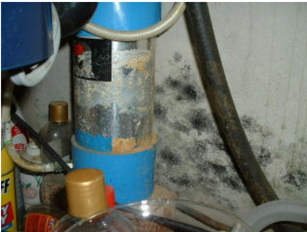
Moisture/Mold damage at wall under Kitchen sink.
