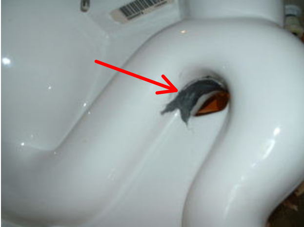
Rear of toilet trap was cracked and patched by "someone" with some type of epoxy. It was leaking at time of inspection.
