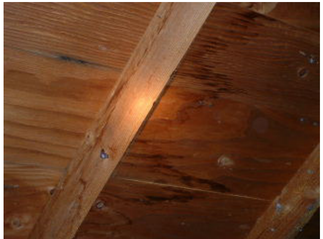
Water damage at under side of plywood roof sheathing due to roof leaks.
