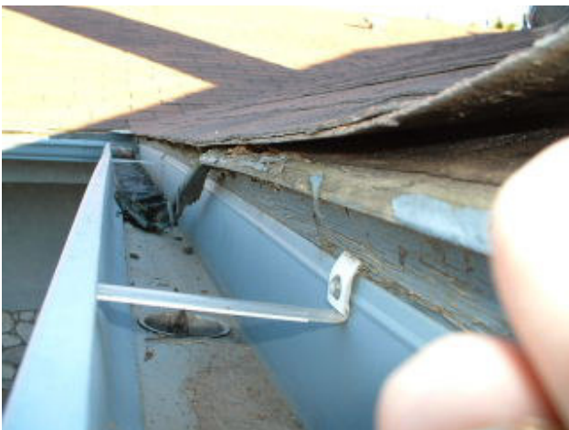
Improper installation of roof underlayment paper; felt paper does not extend out over edges of roof sheathing. This resulted in wood rot.
