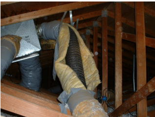
Damaged ductwork in attic common to ductwork manufactured at this time, particularly when exposed to sunlight through attic vents.
