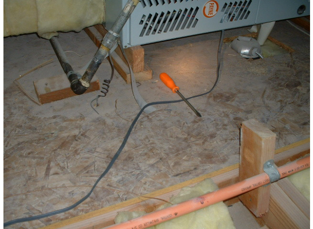
Improper access/clearance at furnace. Requires 30" deep floor (Screwdriver is 10"). Gas pipe, power cord & Fire sprinkler pipe are in the way & subject to damage.
