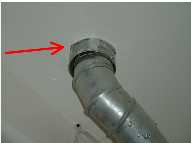
3 year old house: No firestop bucket/thimble installed for water heater vent at garage ceiling penetration. Fire safety concern.
