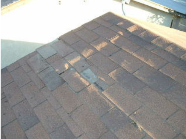
Damaged roof shingles. Improper roof shingle installation; improper overlapping. Improper layout.
