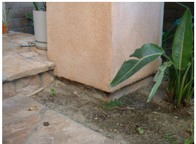
Stoop was built up over weep screed. Sprinkler spray on structure. Resulting in corroded weep screed. Eventual replacement will be needed.
