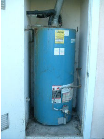
Improperly installed water heater. No seismic straps. Old brackets screwed to top of tank. No overflow pan. Corroded, leaking tank.
