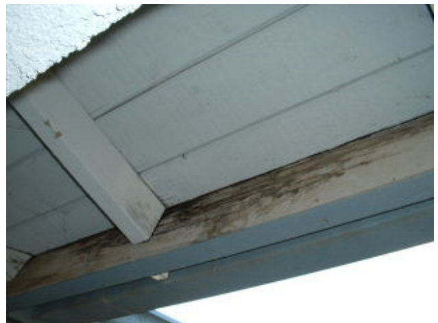
At underside of roof eave, the fascia board was damaged due to improperly installed underlayment paper
