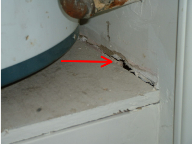
Gap between water heater platform and firewall of garage. Breach in firewall.
