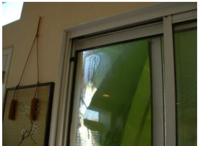
Failed thermal window has condensation between panes and needs to be replaced.
