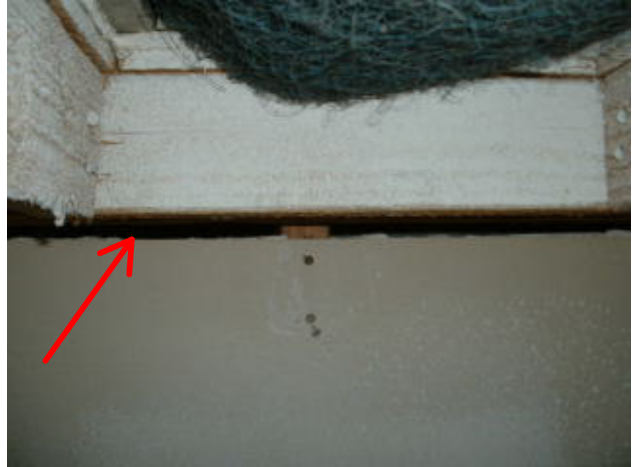
Open gap at plenum wall, under furnace.
