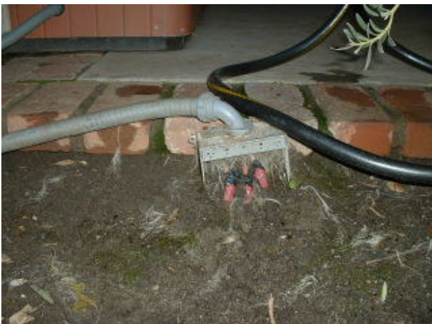
Electrical junction box for Spa was missing cover and was buried in soil.
