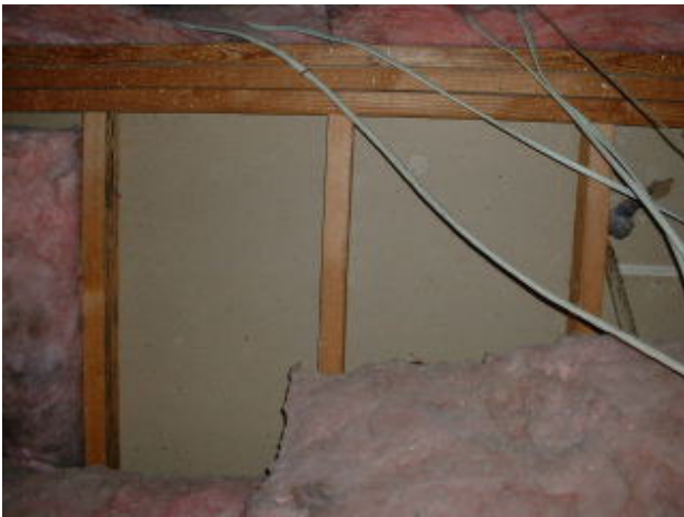
Insulation has fallen down from interior walls in attic.
