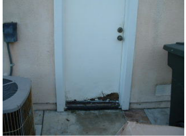
Electrical disconnect box improperly located behind A/C condenser unit. // Excessive wood decay to exterior service door of garage. // Good clearance from weep screed.
