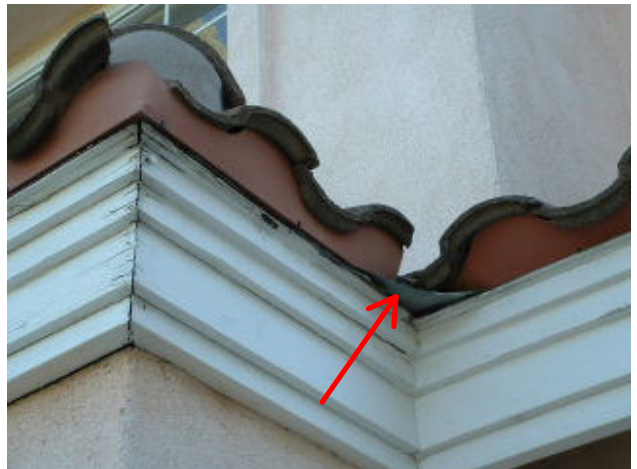
15 year old house: Valley flashing is 16" wide and should fully extend out from under roof tiles. Note resulting water damage at fascia at left side corner.
