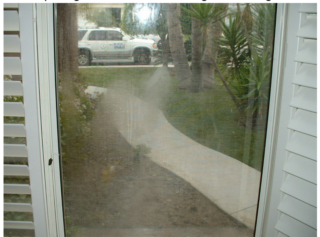
Failed thermal window has condensation between panes and needs to be replaced.
