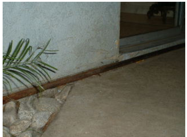
Auxiliary Gas pipe not elevated at least 6" above grade. Also, inappropriately installed under weep screed of stucco siding. Also, in front of toe kick at patio door.
