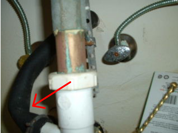
Air conditioner condensate drain hose is kinked under sink. Drainage was blocked.
