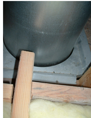
3 year old house: Improper installation and/or fit of the firestop at the fireplace flue as viewed in attic.
