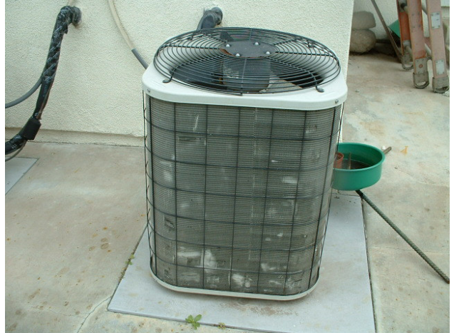
AC compressor/condenser unit is not elevated 3" above finished grade level and not secured in place. Dented heat dissipating fins. Fins are starting to disintegrate.
