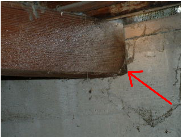
No Beam pocket molded into foundation wall. A main beam was left unsupported and not stabilized at this end.
